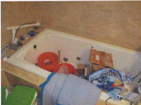
Bathtub is inoperable
