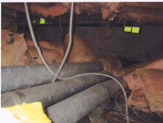
Heating ductwork just laying on vapor barrier
