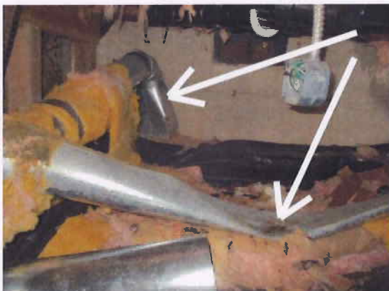
Crushed ductwork, disconnected ductwork
