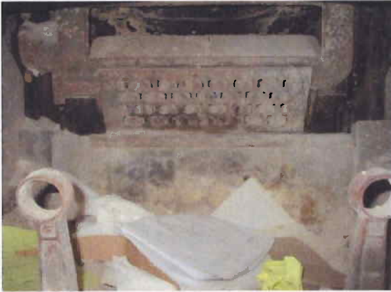
Woodstove cleaning recommended
