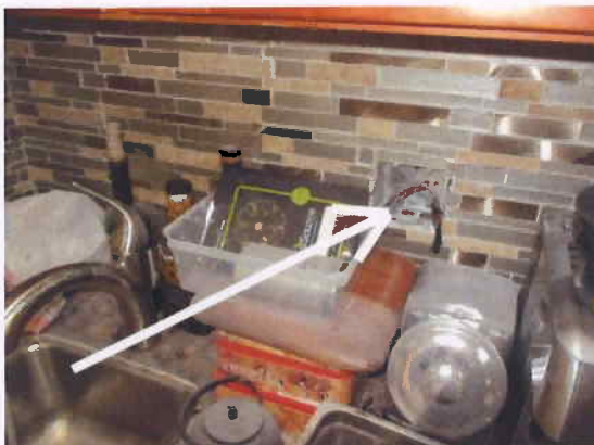
Wiring hanging out of junction boxes at the backsplash in the kitchen
