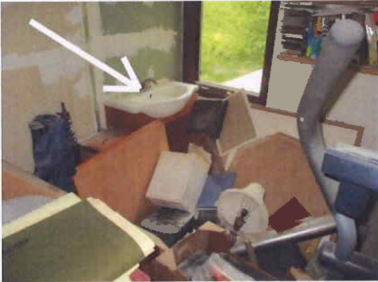
Could not access this sink
