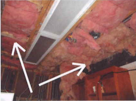
It looks like rodents are nesting in the garage ceiling insulation
