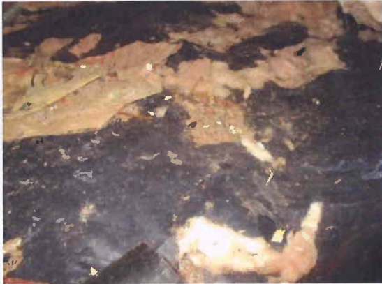
Rodent contaminated vapor barrier
