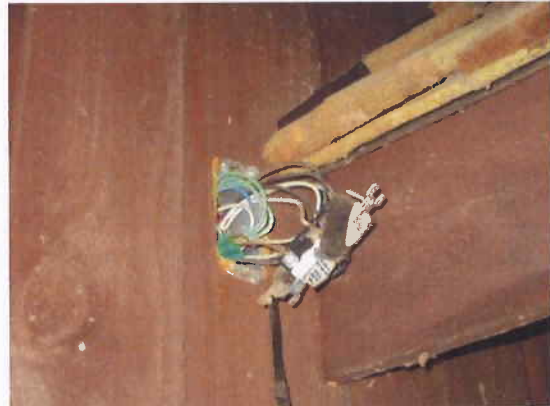
Lots of loose receptacles
