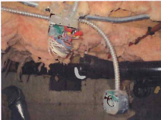
Lots of exposed wiring and loose junction boxes in the crawl space
