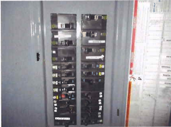
Main panel - nearly half of the circuit breakers are shut off
