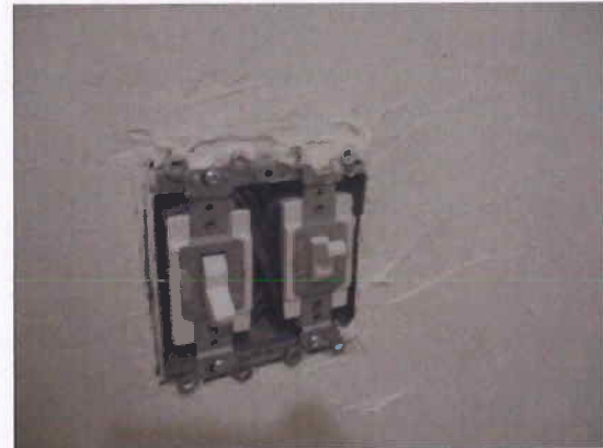
Most switches are missing cover plates
