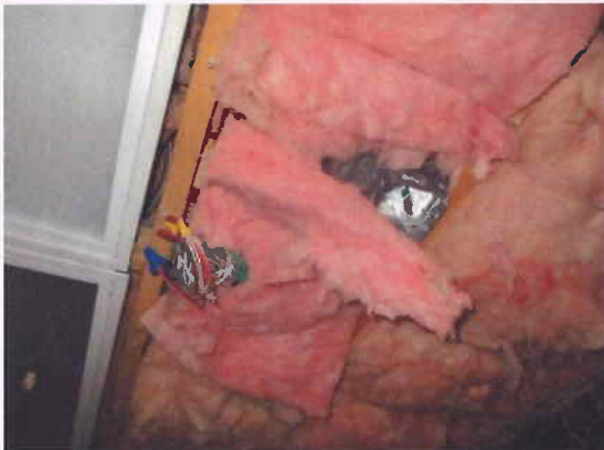
Garage ceiling has no firewall
