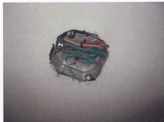
Many uncovered junction boxes throughout the house
