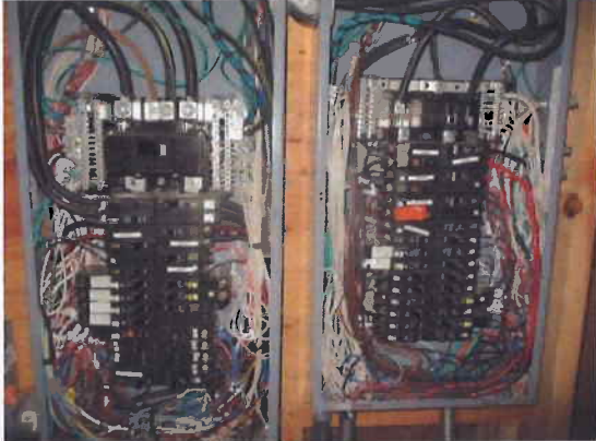
Main panel (left) and sub-panel (right)
