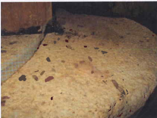
Rodent feces in crawl space
